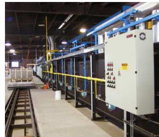
Gas fired car tunnel kiln for traditional ceramics
